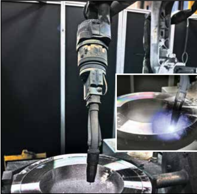
Automatic plasma arc hardfacing equipment of a wedge using a robotic arm.
