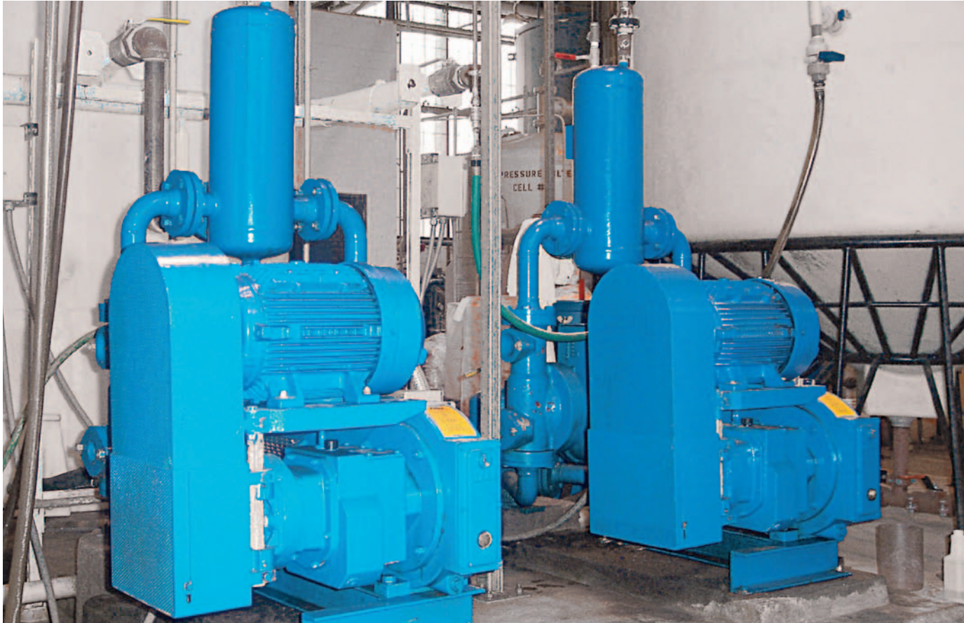
ABEL HMD-G-12-0060 for transfer of contaminated sludge from soil washing process
