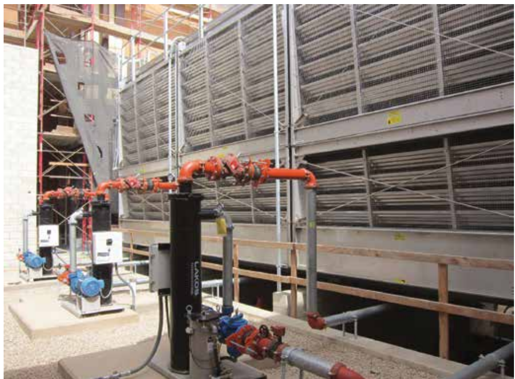
LAKOS HTX Separators on packaged TCX systems keep this cooling tower clean at a Resort and Spa in Hawaii
