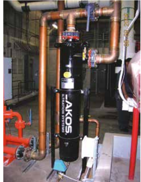
HTX used to prevent sand from entering toilets and other water supplies at large Convention Center in Florida
