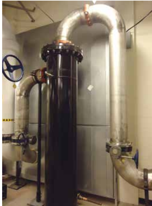
HTX installed at Peppermill Casino in Reno, Nevada, keeps their geothermal heat exchanger clean and free of dirt. The Peppermill has won numerous awards for its facility, including Green Company of the Year
