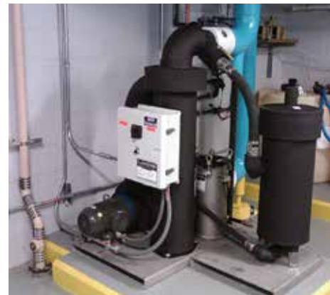
Closed loop Filtration, Data Center, Virginia USA
