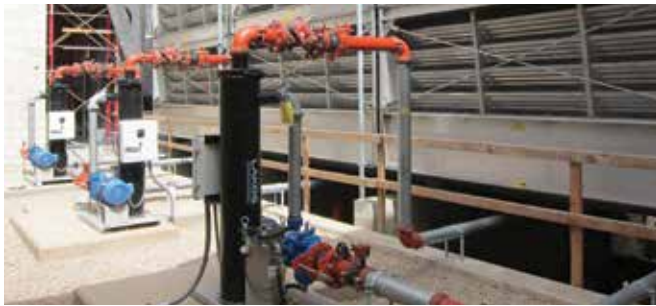
TC Systems in Aulani Disney Hawaii Resort, Hawaii USA
