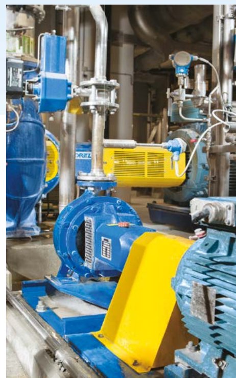
Installed ANDRITZ pumps ISO series
